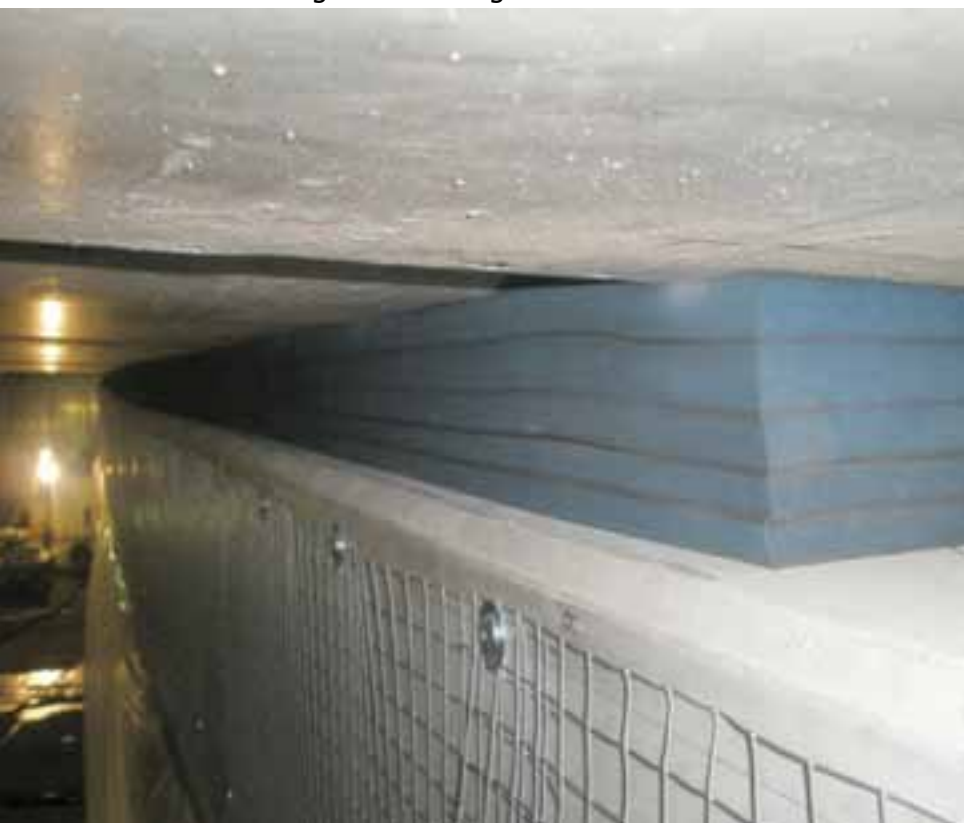
The new retardant material sandwiched between ceiling and wall in the Victoria Park tunnel. Photo: CSD.
