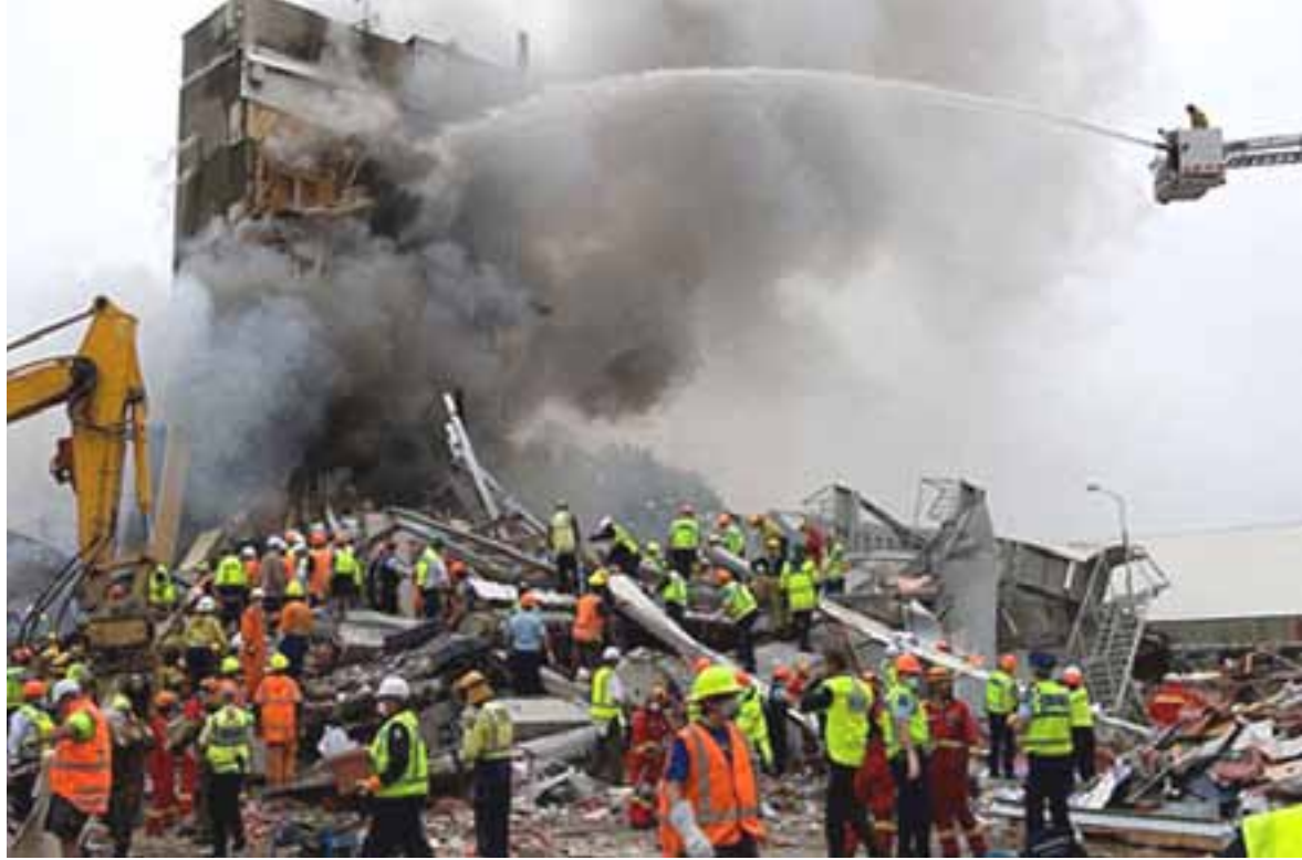
Firefighters, police, council and construction workers pour over the collapsed CTV building in Christchurch.
